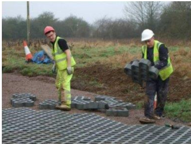
Easily handled interlocking blocks rapidly placed across the prepared surface, leaving a flush surface allowing heavy vehicles to turn without causing drag on the blocks
