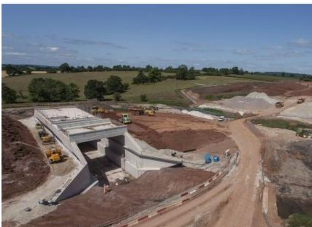
Using Deckdrain drastically reduced the number of vehicle movements on this busy site
