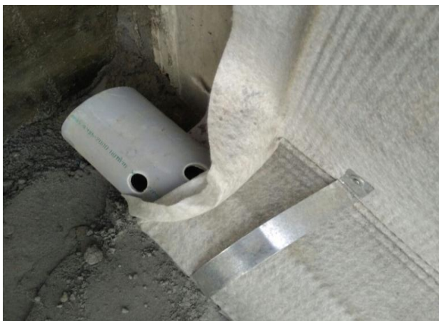
ABG Deckdrain secured and wrapped around the perforated drainage pipe at the lower end
