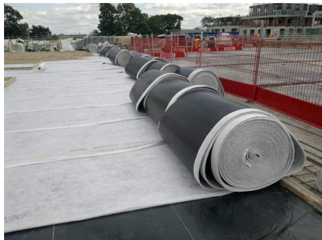
Small rolls of Deckdrain are quickly laid directly on the waterproofing on the concrete roof slab and walls.
