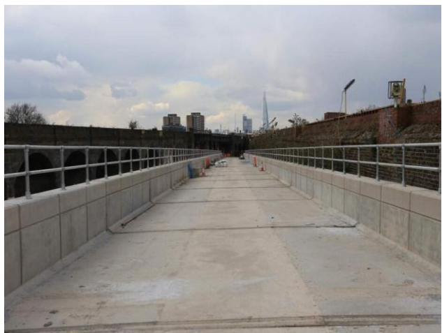
Finished deck ready to receive trackbed separated from restored arched railway viaduct
