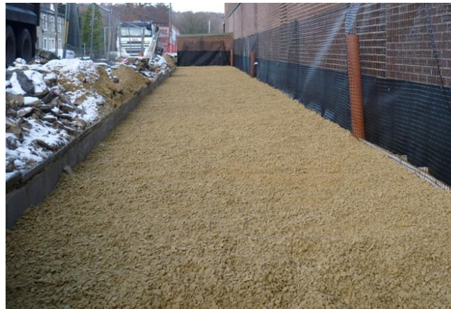
Trigrid temporarily held against brick wall as crush stone fill is placed.
