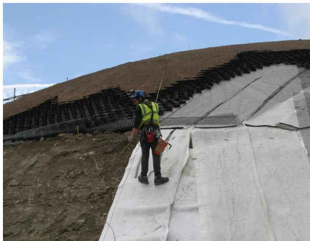
Geogreen Solutions working from harnesses to install the three layers bolting them to the timber structure to provide a stable surface to encourage growth
