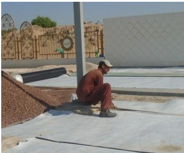
Installing the Pozibreak ensuring the overlaps of filter geotextile prevent cover soil entering the capillary break void and causing tracking
