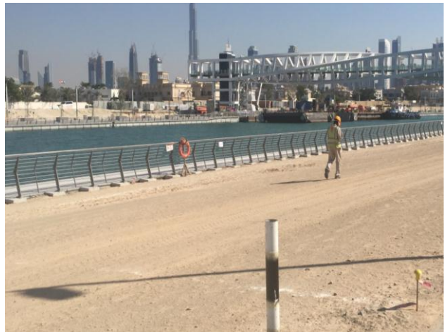
ABG Salt Barrier installed underneath landscaping running along the side of the canal
