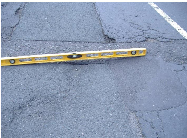
Stressed road surface needing re-surfacing late 2010
