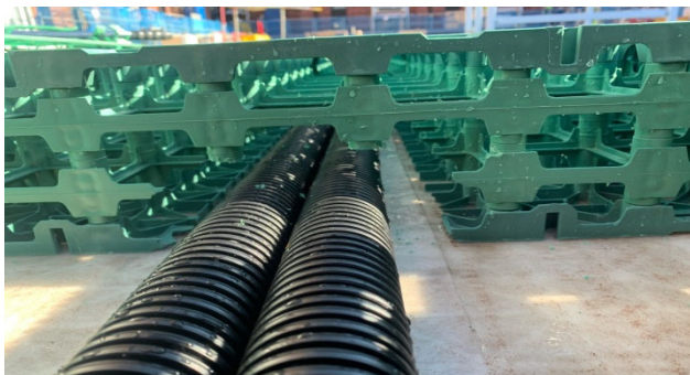
Cable ducting routed through the attenuation voids
