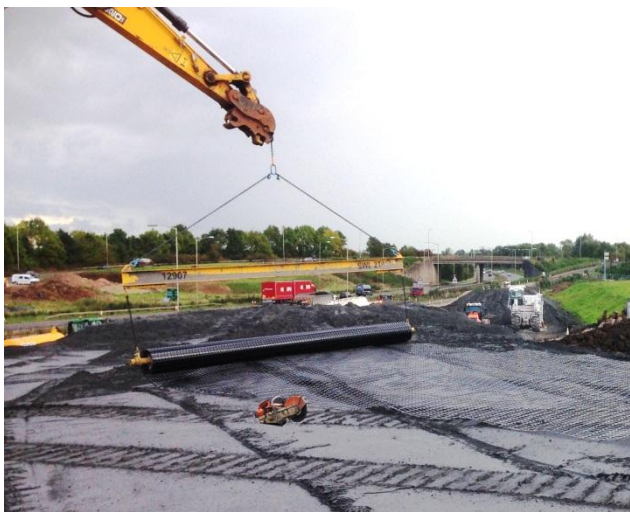
Spreader beam used to position grid and cut to suit using a disk cutter
