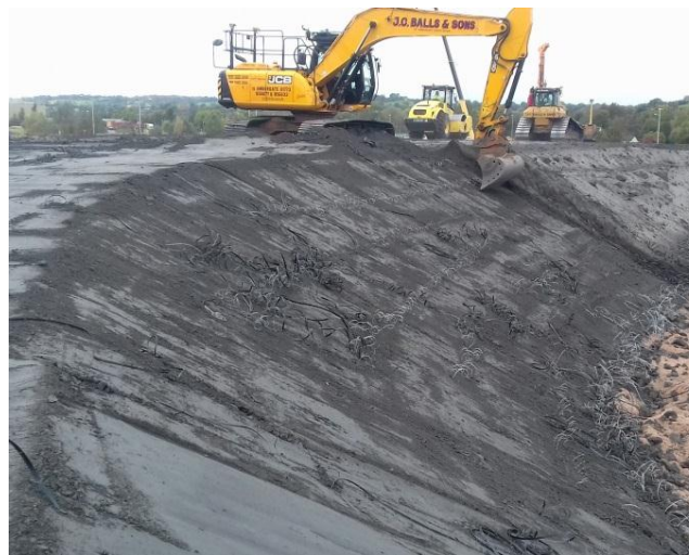
Trimming of the embankment through the compacted reinforced slope ready to receive topsoil
