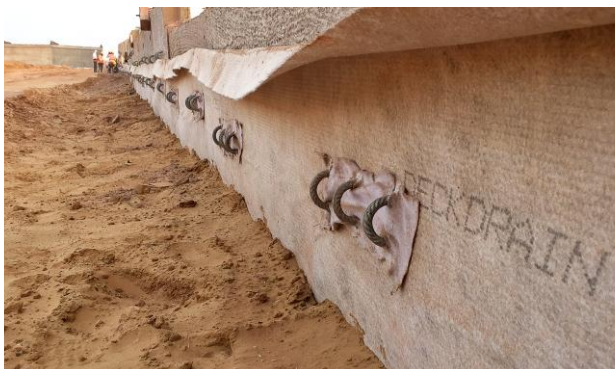
Hook bars from the RE panels carefully pierced through Deckdrain and later made good with geotextile
