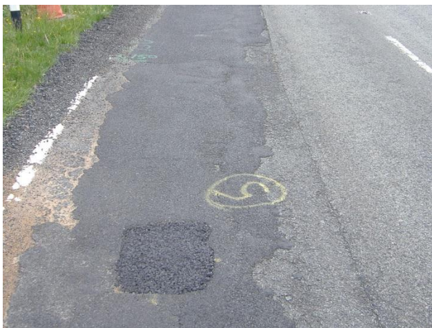
Previous multiple attempts to patch the road edge
