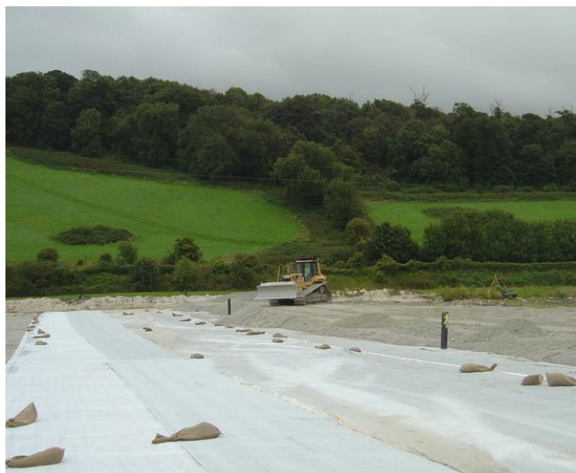
Adequate interface friction ensured slope stability
