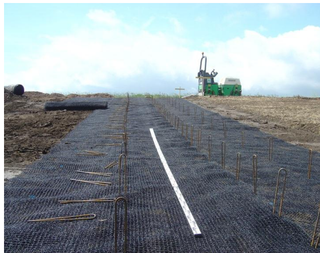
Correct surface preparation and pinning are essential to maintain good surface contact with the underlying soil followed by careful seeding and filling.
